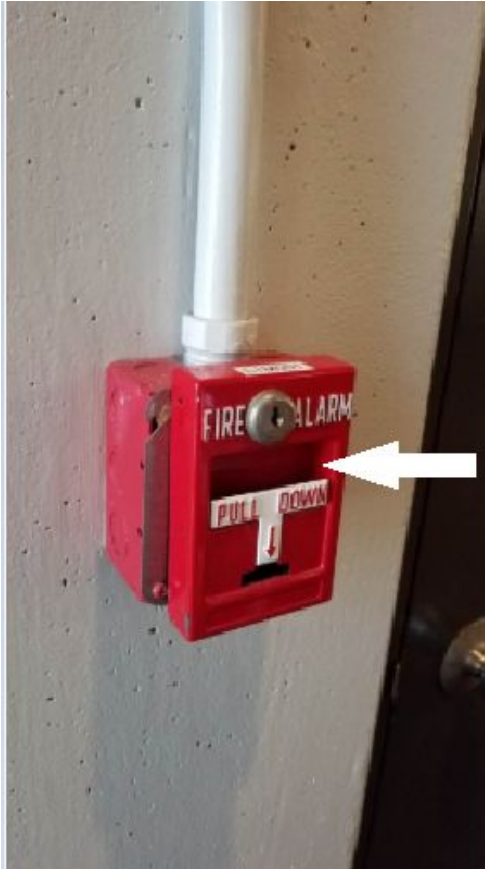
Figure 1A: An up-close look at the fire alarm inside Mandeville Auditorium. It is considered a good design due to the clearly marked lever and function.
